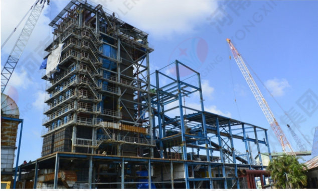
2017.08 新疆乌鲁木齐宝塔石化50吨循环流化床锅炉 2017.08 50t/h CFB boiler in Wulumuqi Baota Petrochemical Co.,Ltd
